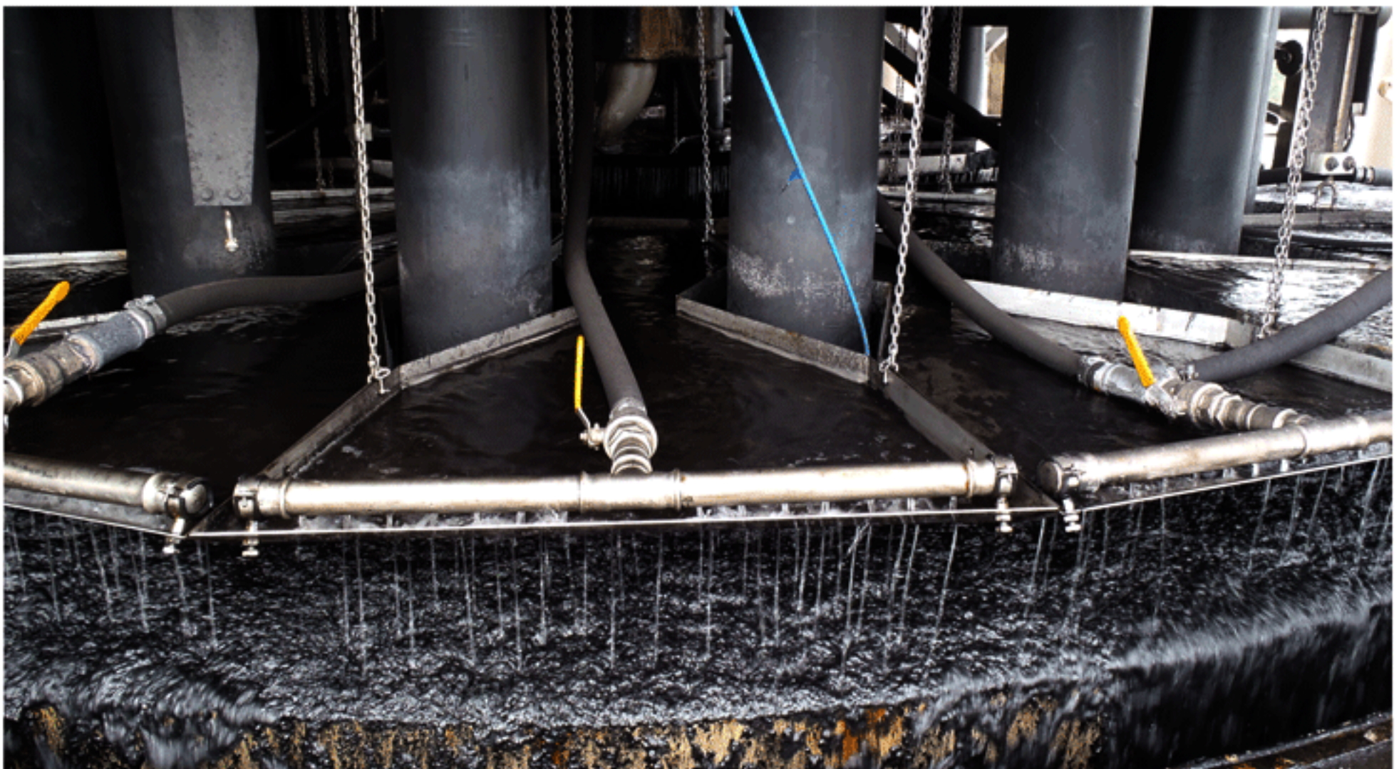
CleanProTech froth washing system installed on a Jameson flotation cell.
